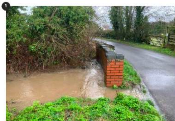
Figure 56: Flooding on Common Piece Lane on 18th February 2024. Common Piece Lane is a rural road, which is not a through way for road traffic, but is a vital route for access to farming land, and a pleasant green walking route which provides connectivity between the village and residential areas, conservation areas around Cardale's Meadow, and the Trent and Mersey Canal.
