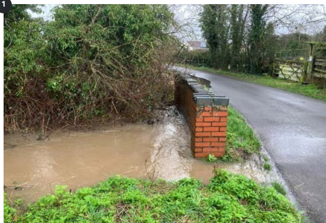
Figure 56: Flooding on Common Piece Lane on 18th February 2024. Common Piece Lane is a rural road, which is not a through way for road traffic, but is a vital route for access to farming land, and a pleasant green walking route which provides connectivity between the village and residential areas, conservation areas around Cardale's Meadow, and the Trent and Mersey Canal.
