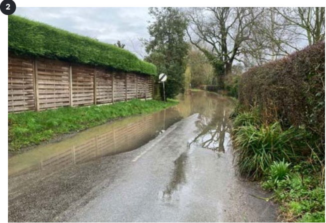
Figure 57: Flooding on Bakeacre Lane on 18th February 2024. An essential transport route providing key links to local schools.
